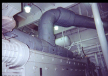
Manifold, Exhaust & Expansion Joint
