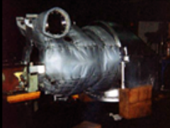
Elliott Compressor After
